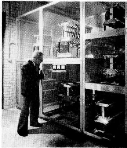
150kW ATH with additional rejectors, covers removed.
